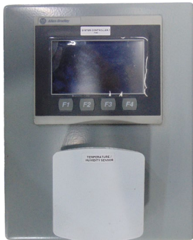
WALL MOUNTED CONTROL PANEL WITH HMI AND TEMPERATURE SENSOR
